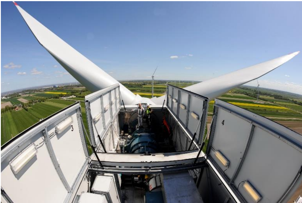
Figure 1 PNE technical staff in a turbine nacelle, 2017
